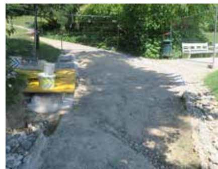
Fig. 98 The maintenance of the Kurgardens is never ending. Reconstruction works on the parkway sewage system in 2019.
